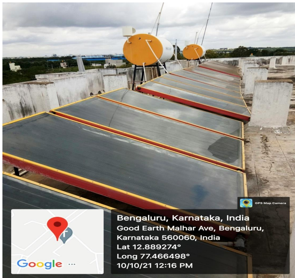
Photo: Solar Panels for water heating
