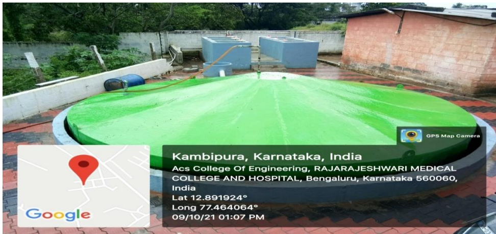
Photo: View of the new Biogas Plant at ACSCE
