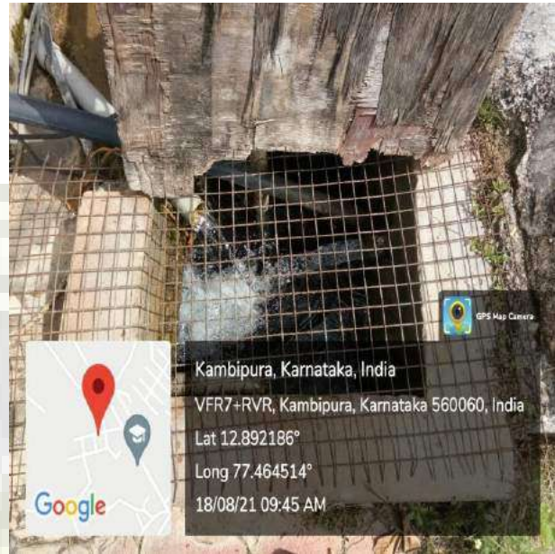
Photo: Underground water Storage Tank in the Campus
