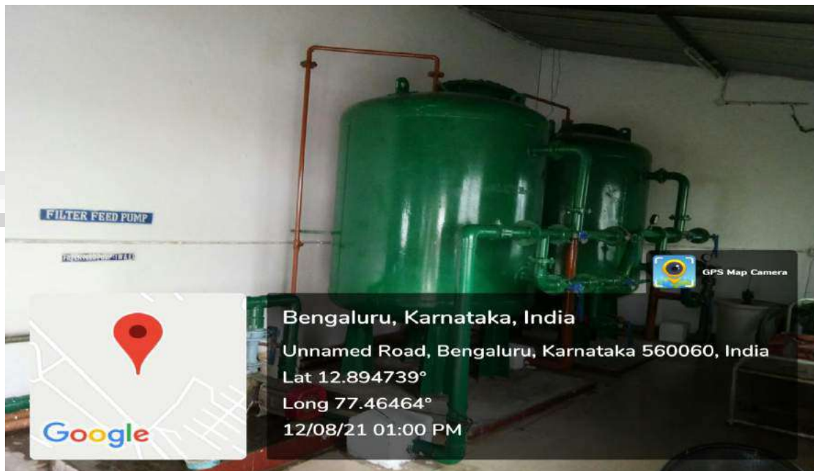
Photo: Sewage Treatment Plant of 300 KLD in operation
