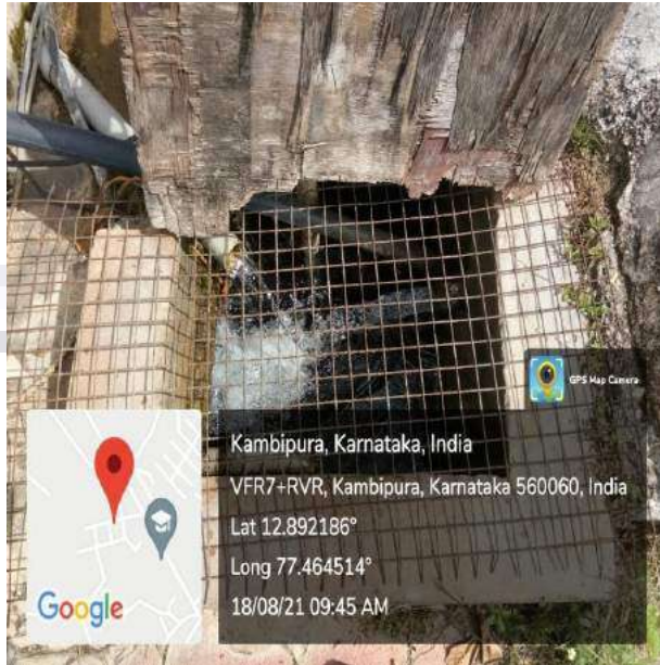
Photo: Over Head Tank in the campus building
