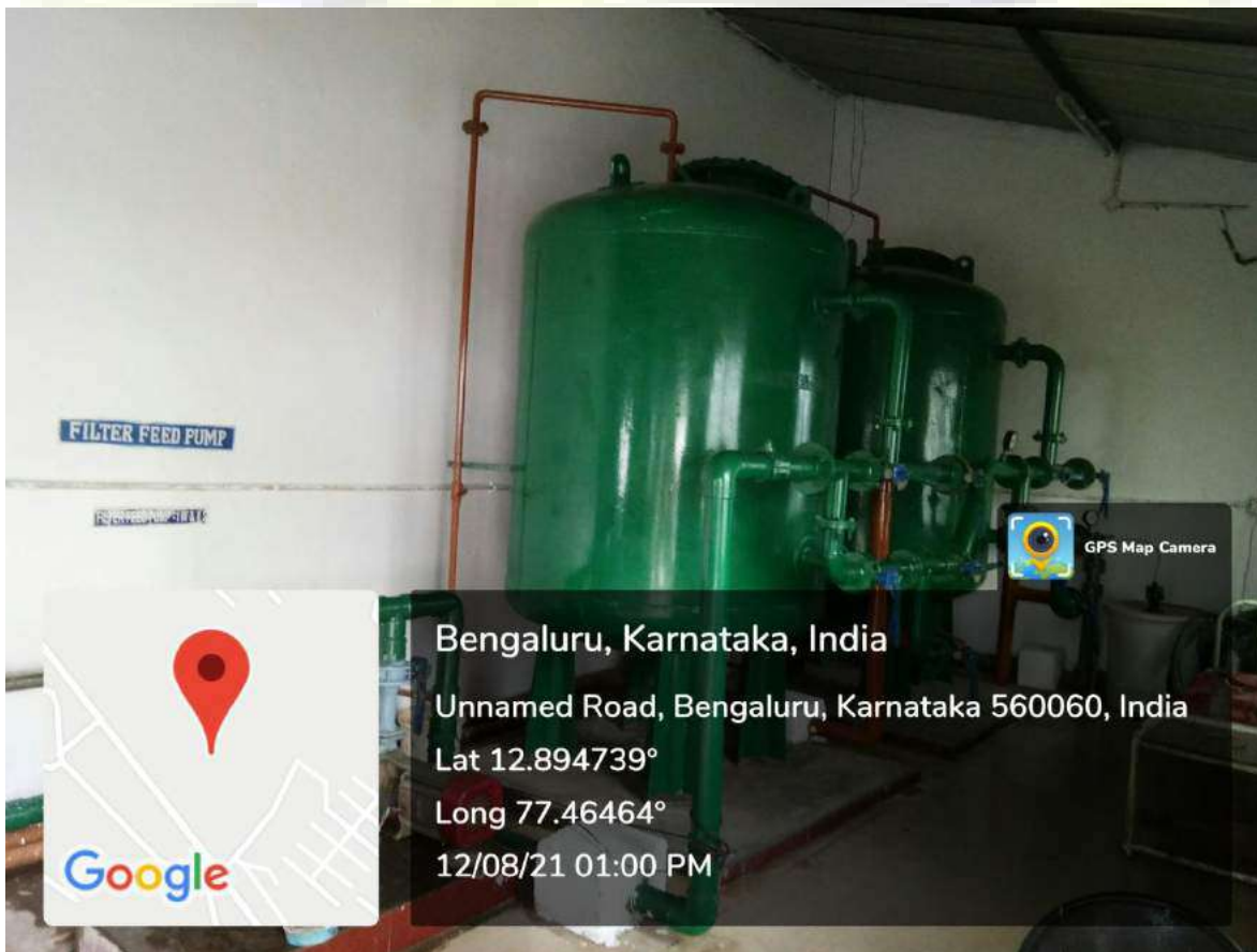
Photo: Sewage Treatment Plant in operation
